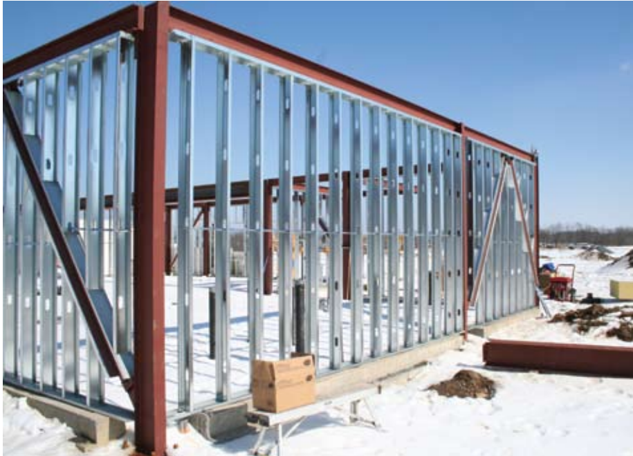
PC Haines project site, Area 6, Fort Indiantown Gap, PA, steel stud installation.
